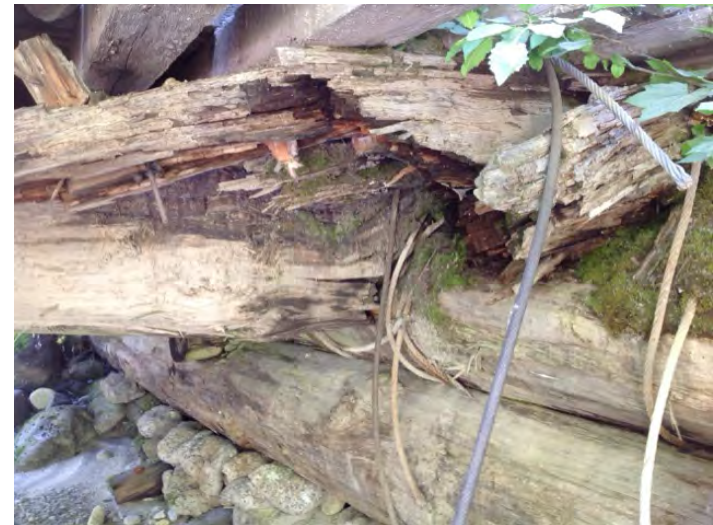
downstream log stringer, left side completely sheared
