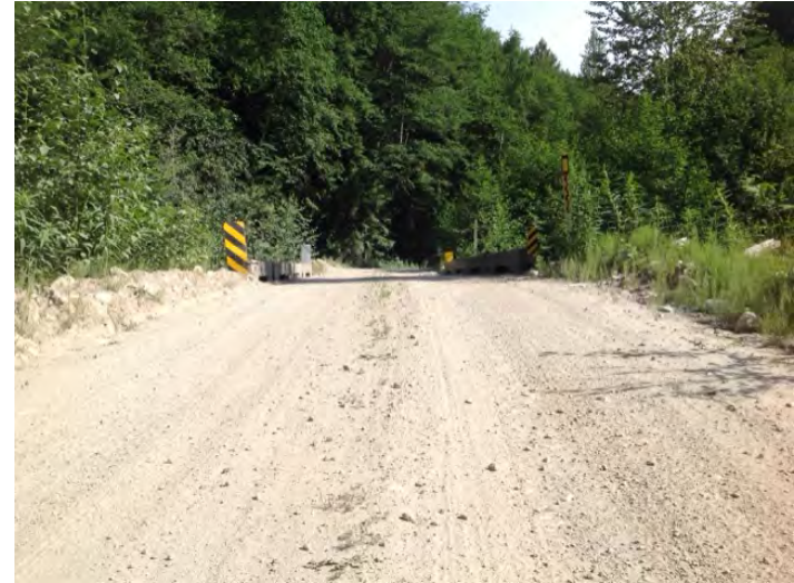
structure appears to be settling on downstream end
